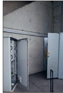
Abb. 4: Standort Outdoor-System an Tunneleingang
